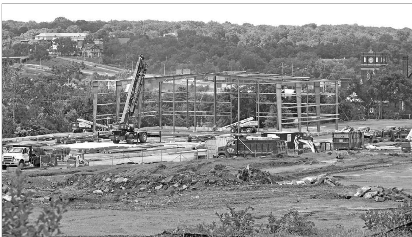
Construction on the East Side chill-can plant is ahead of schedule. The site on North Lane Avenue will have multiple production buildings and will be the East Coast headquarters for Joseph Co. International.
