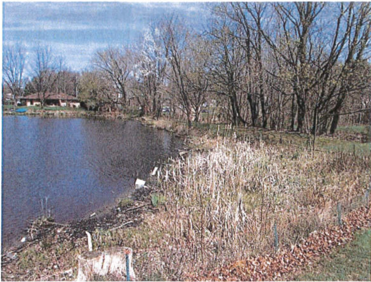
Photograph No. 1: View of the upstream slope from the right abutment. Note the tall vegetation growing on the slope.
