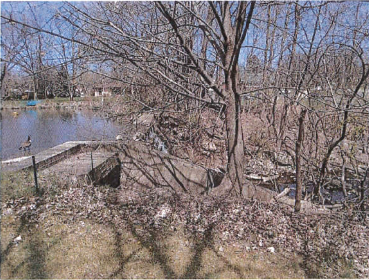
Photograph No. 5: View of the downstream slope from the left end of the dam.
