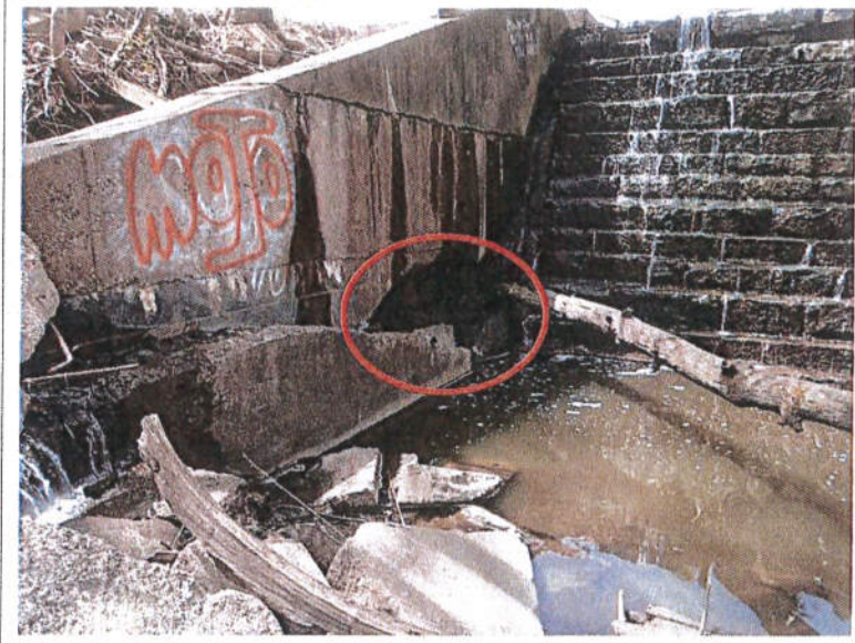
Photograph No. 10: Another view of the left sidewall. Note the severe damage to the concrete.
