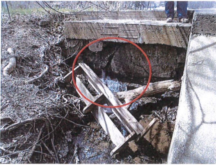
Photograph No. 8: View behind the left sidewall of the principal spillway. Note the large crack in the concrete and the large amounts of water seeping through.
