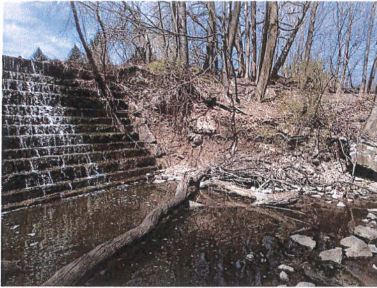
Photograph No. 7: View of the principal spillway. Note the right sidewall has collapsed and has been washed downstream.
