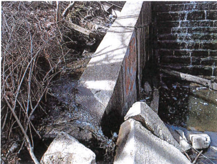
Photograph No. 9: View of the left sidewall. The water leaking from the crack in the picture above is eroding the soil behind the sidewall and seeping through cracks in the sidewall.
