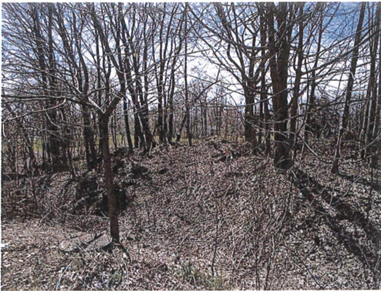
Photograph No. 4: View of the downstream slope from the left end of the dam. Note the trees and brush on the slope.
