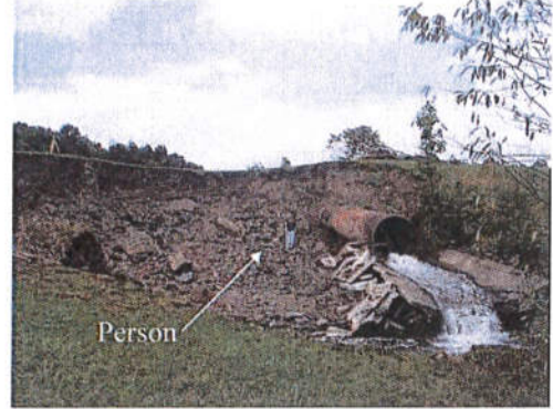
Erosion caused by floodwater overtopping the dam – a result of inadequate discharge/storage capacity and debris obstructing the 5-foot-diameter spillway pipe.
